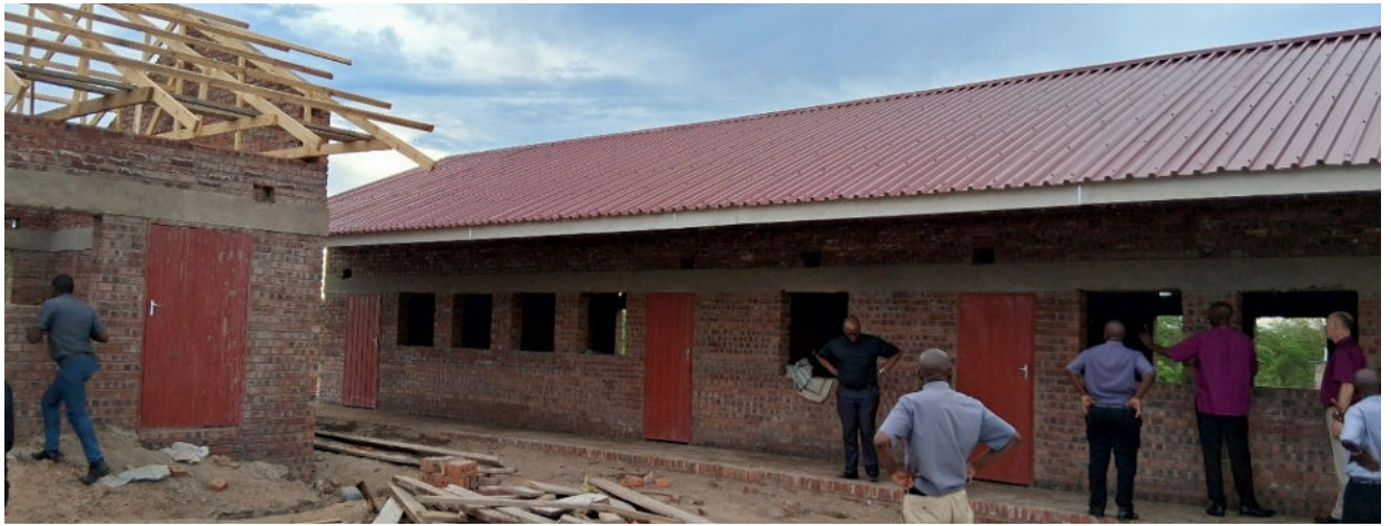
Two classroom blocks at the roofing stage, at St Cecilia Mission, Lupane.
