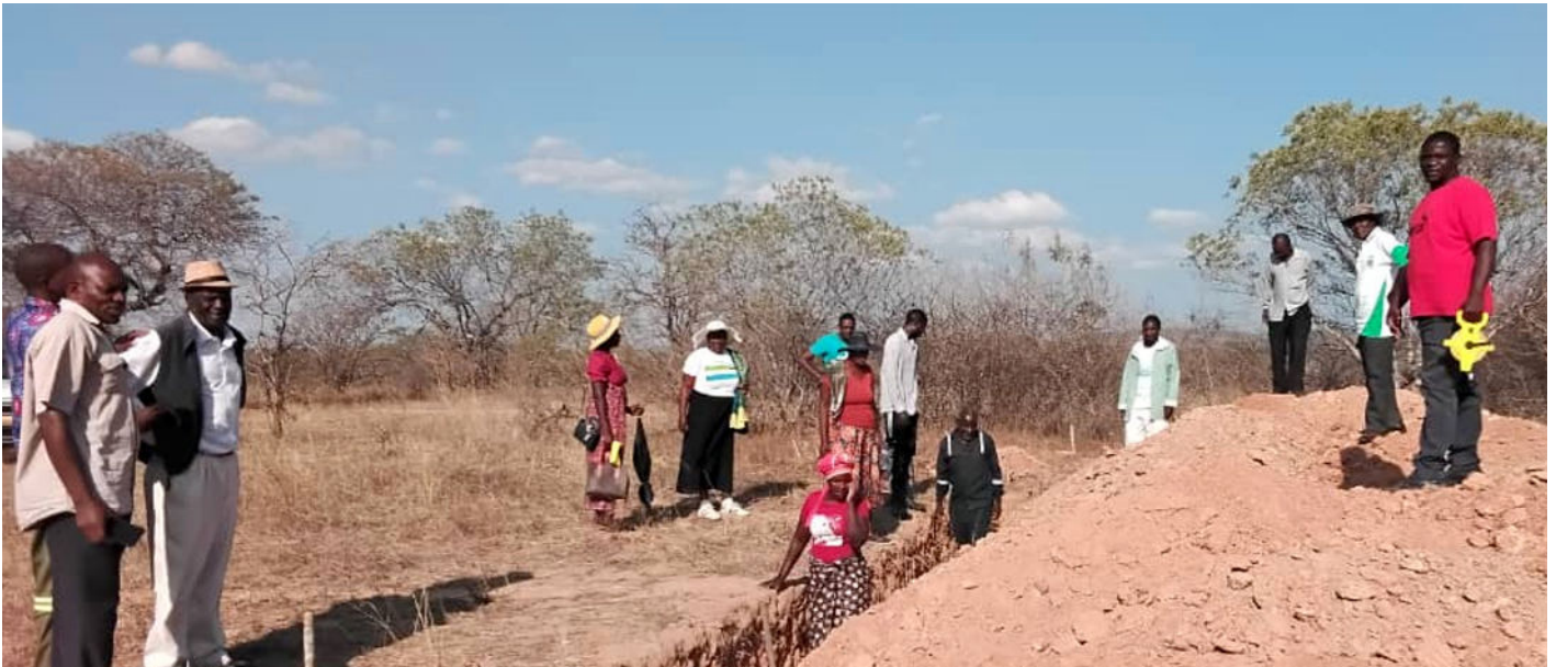
St Mark's Mission, Filabusi baptism candidates and members of the community digging the foundations for the chapel.
